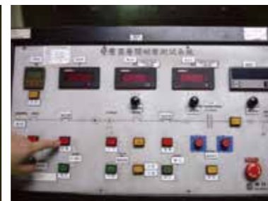
感應電壓測試 Induced AC withstand voltage testing
